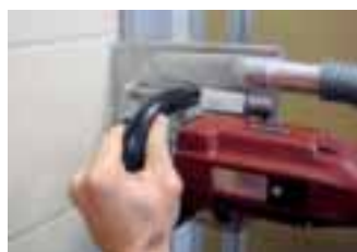
Cut into the tiled wall
