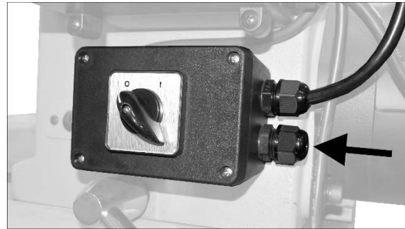
Figure 7-1: main switch box
